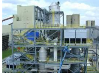
AEP Mountaineer USA - 58 MWth Chilled Ammonia - Coal
