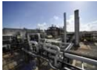
Total Lacq France - 30 MWth Oxy - Gas
